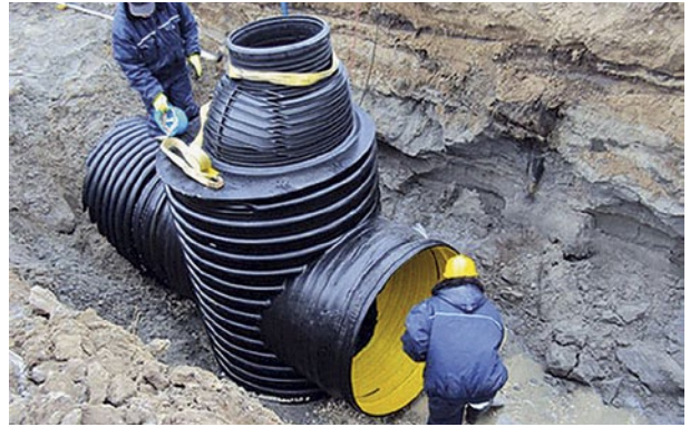
Inspection manhole for rainwater DN/ID1500
