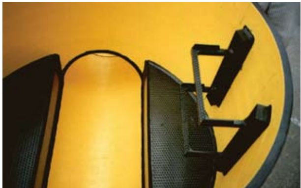
Inside of a standard manhole with a berm and stairs
