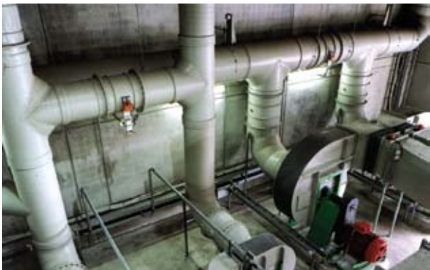
Industrial ventilation pipes
