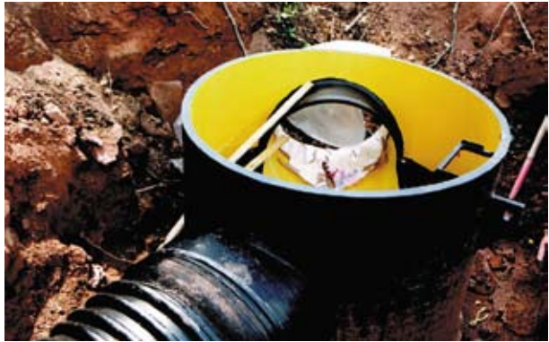
Standard manhole DN/ID 1000mm
