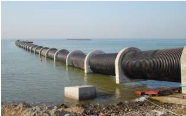
Sea outfall pipe line DN/ID 1800mm
