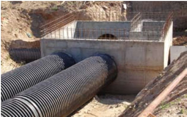
Main collector of a sewage treatment plant
