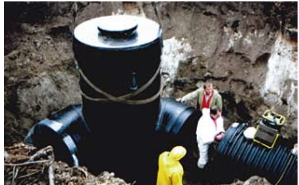
Manhole with an integrated bend and electro fusion joint
