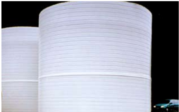
Vertical "stepped" storage tank for industrial applications
