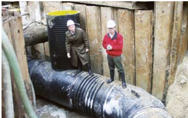
Sewer line DN/ID 1200mm with bend and manhole jointed by electro fusion
