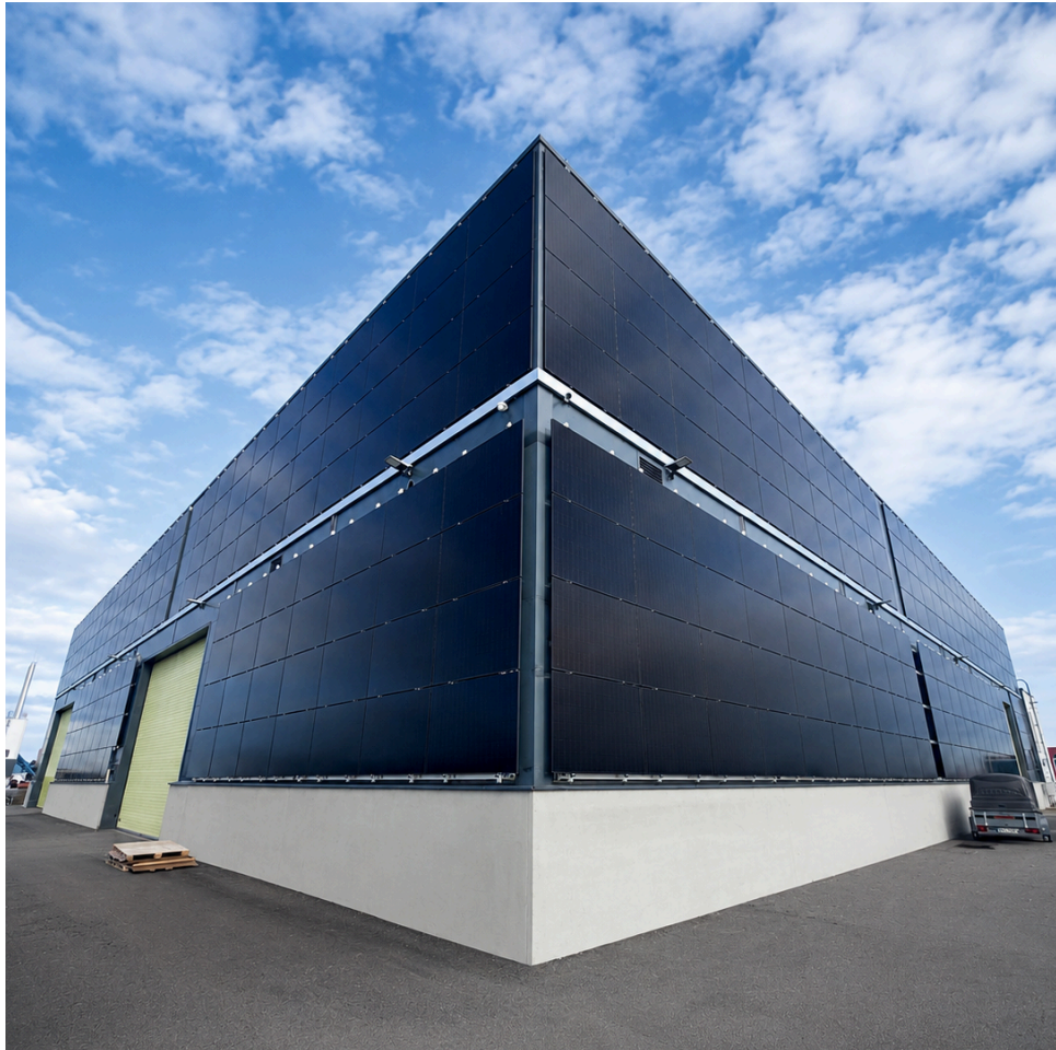
Solar PV installation at Krah Pipes facility in Lehmja, capacity expanded ~84% in 2025
